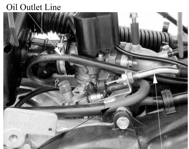
Oil Inlet Line
