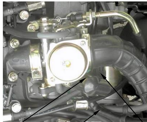
Earth Cable Fuel tube Starter Motor Cable
